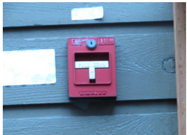
Fire Alarm-Pull Station
